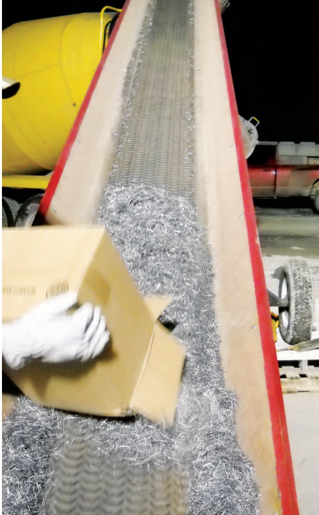
Steel fibers are being loaded into a ready-mix truck. Fibers are usually added at the concrete plant, but can also be added onsite.
